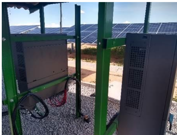
Figure 27 - Power plant PV system and inverters (Source: Lactec).
