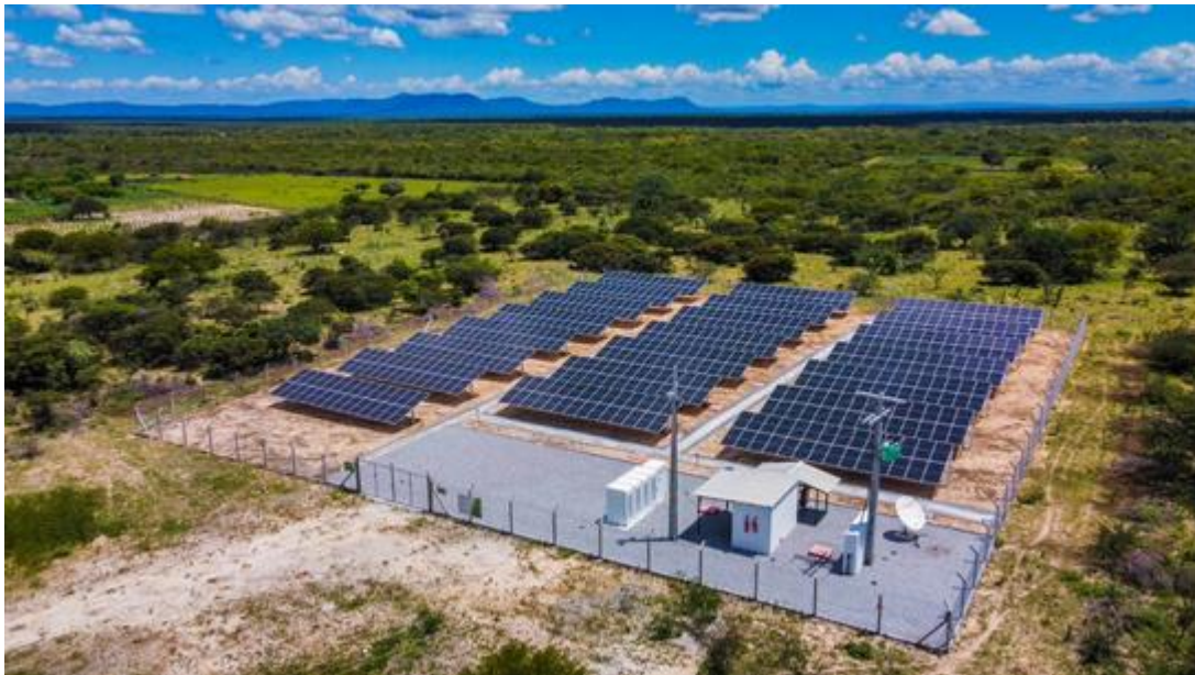
Figure 25 - Aerial photo of the microgrid pilot plant (Source: Neoenergia Coelba).
