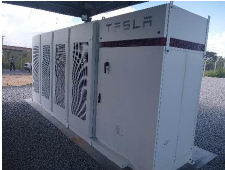
Figure 28 - Power plant BESS (Source: Lactec).
